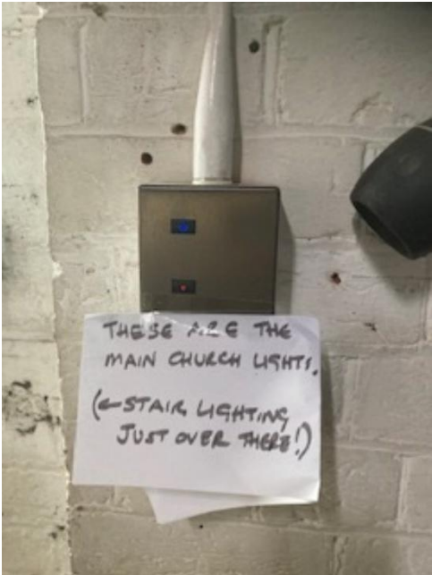
Light switches for church in cupboard found on left of the alter.
